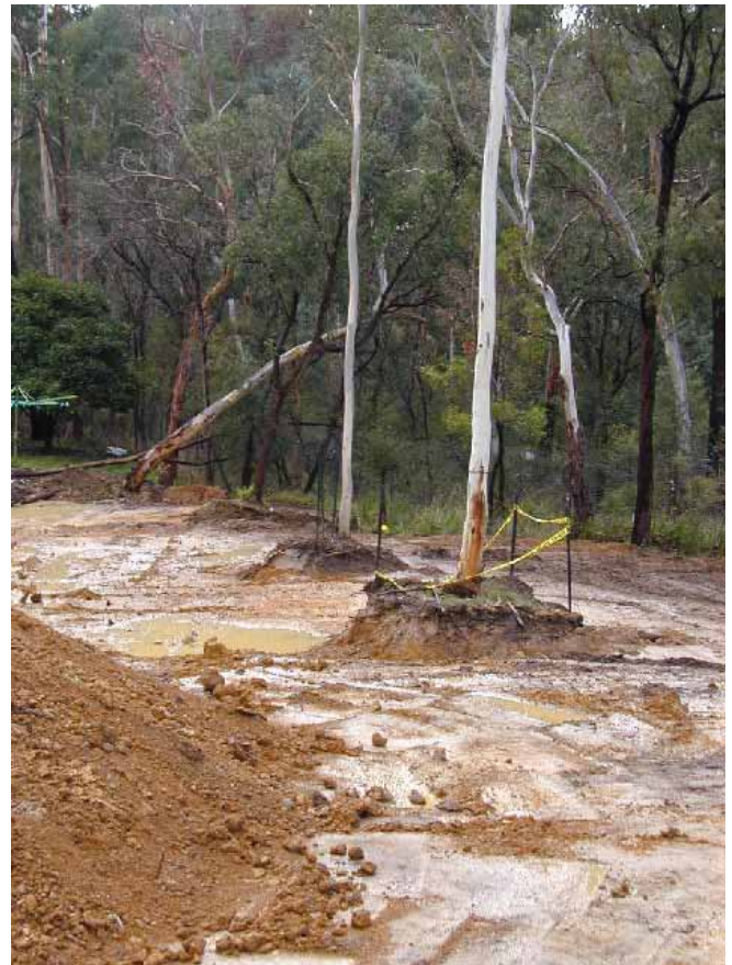
This tree protection zone has not protected the critical root zone. The Candlebark trees will not survive this excavation
