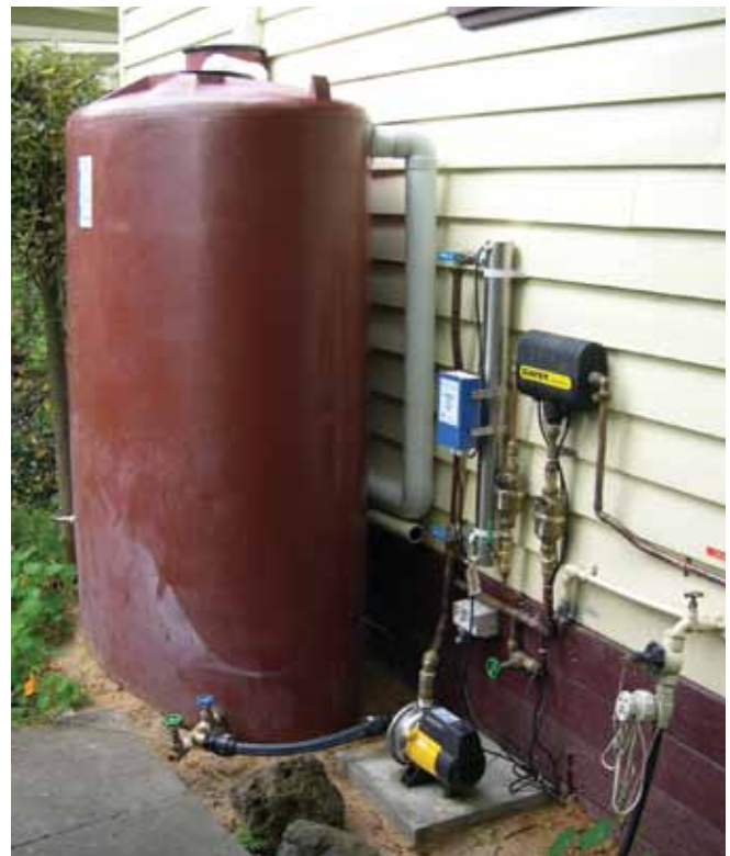
Typical pump control centre for internal house use e.g. toilet and washing machine use
