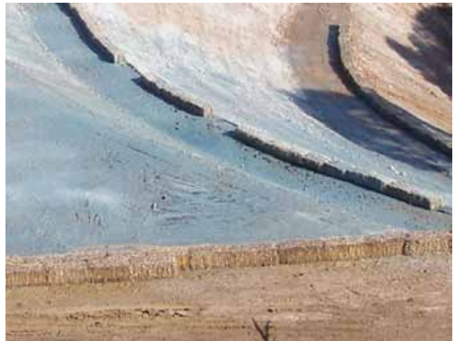
Hydroseeding and hay bales can be used to reduce erosion and runoff
