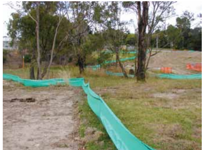
Use sediment fences around the excavation zone to reduce turbidity of waterways
