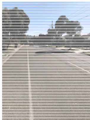
Faded Line Marking – Sheahans Road Manningham
