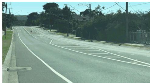
Good Line Marking Blackburn Road Manningham
