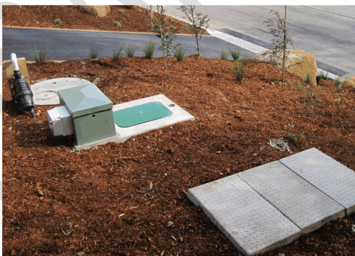
Figure 2: Treatment Plant with sub-surface irrigation
