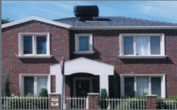
Siting air-conditioning and other plant behind the front roof pitch will improve building appearance.
