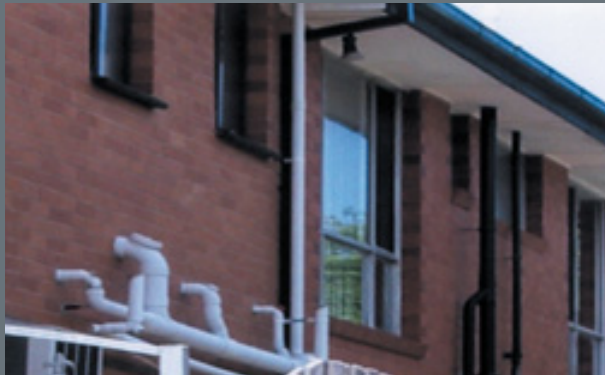
Exposed pipes detract from the appearance of buildings.
