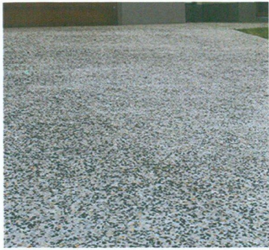
POLISHED EXPOSED AGGREGATE PAVING
