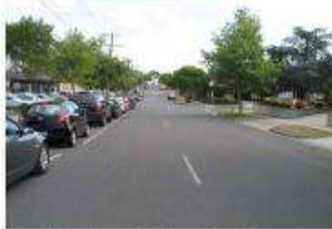
Faded Line Marking - Grant Olsen Avenue
