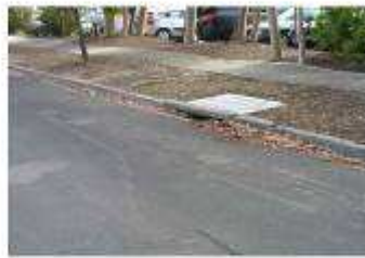
Blocked Pit – Derreck Avenue -
