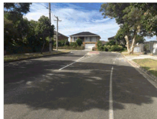
Faded Line Marking - Sheahans Road Manningham
