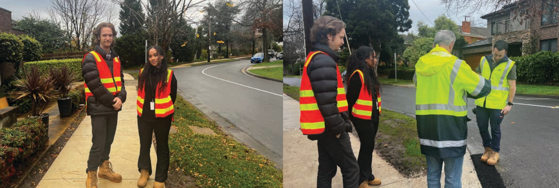
ABOVE: Cadet engineers Hugh Martin and Rochelle Cabral inspecting works in Doncaster.
