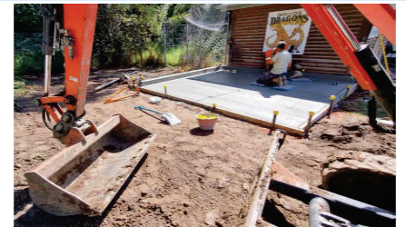
Concrete pad installed for storage of red porous material for the baseball diamond at Deep Creek Reserve
