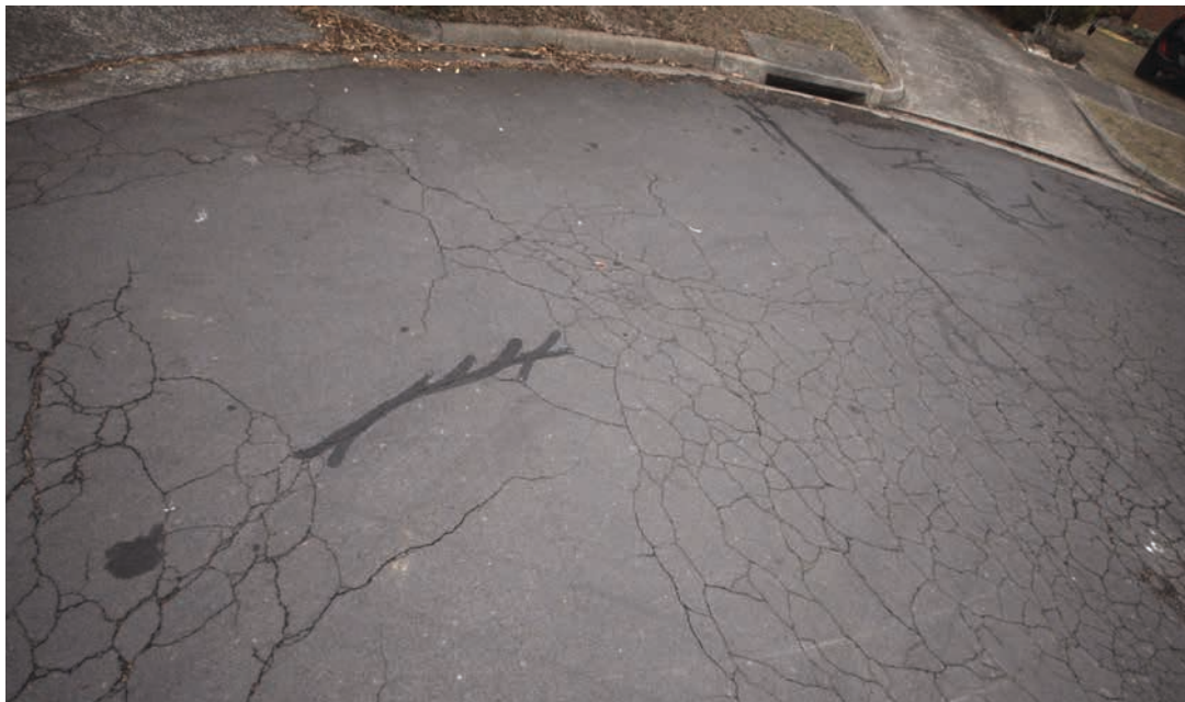
Figure 19 Snapshot of a very poor road surface (Wallmah Close in Templestowe)
