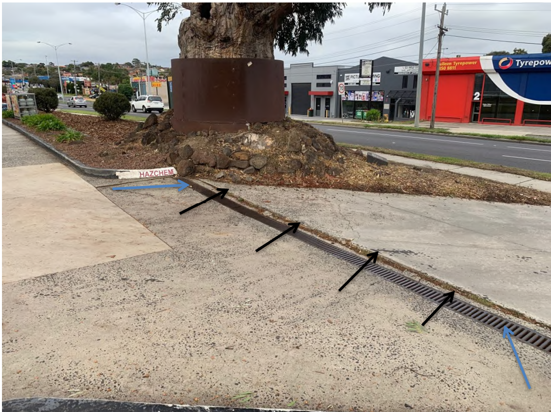
Photo 12 – The black arrows indicate where the slab of the driveway is rising and lipping relative to the metal grid of the drain and the concrete inside the service station. It is probable major root development is occurring beneath the drain, arrowed blue, causing lifting of the drive.
