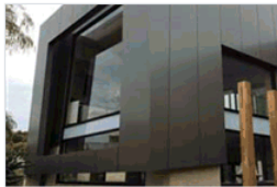
F02 SELECT METAL CLADDING WITH EXPRESSED JOINTS TO EXTERNAL WALL. COLOUR TO BE 'CHARCOAL'.
